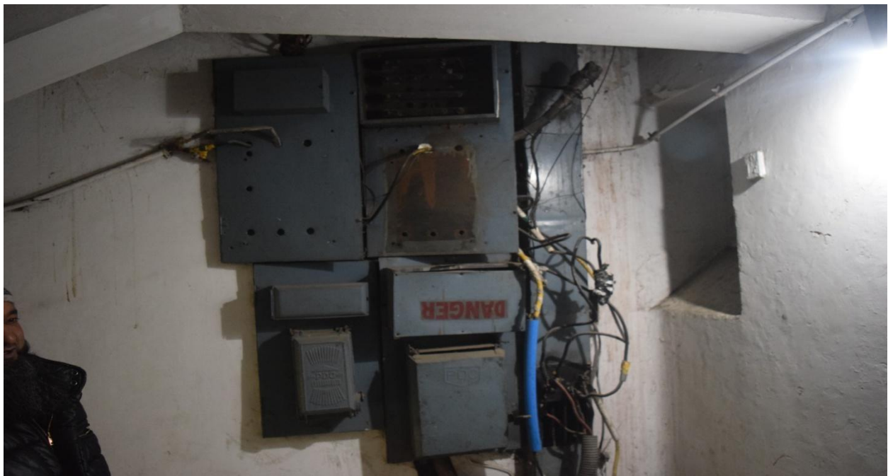
Plate.10. Electric panels posing threat to life
