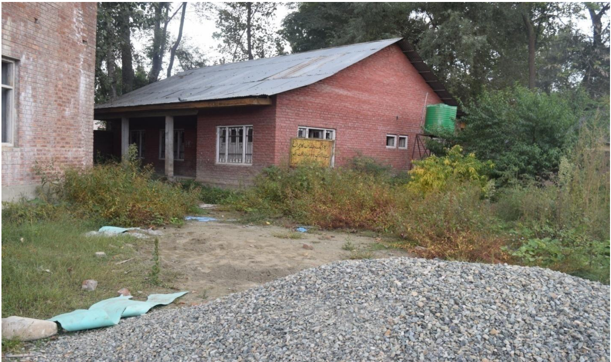
Plate4..flood damaged single story building
