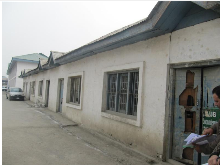
Existing damaged building
