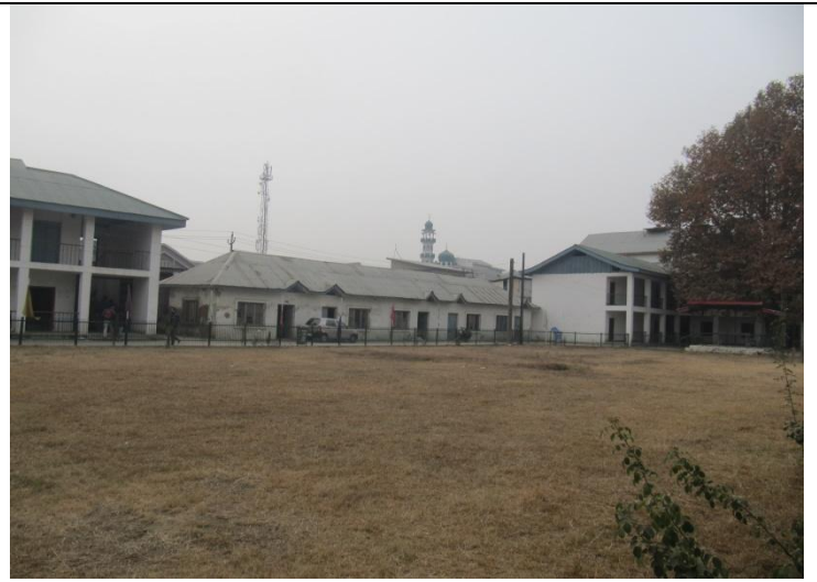
Existing damaged building in school premises
