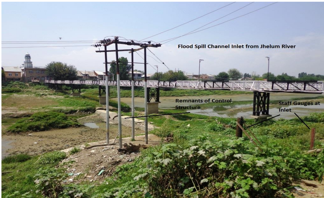
Photograph of Flood Spill Channel Inlet – Remnants of Concrete Control Weir Remains
