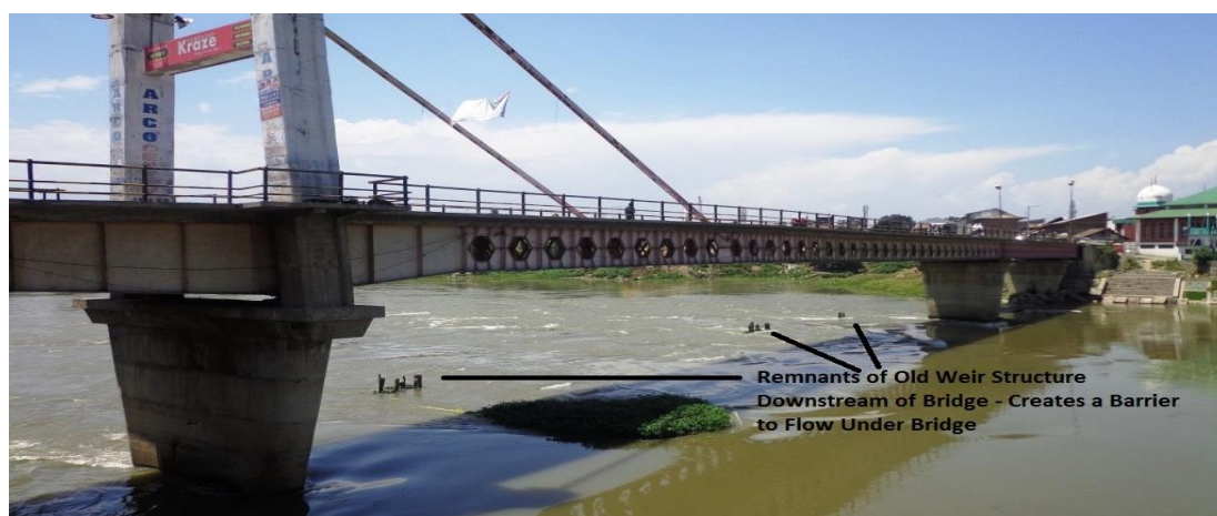
Photograph of a Bridge Structure near Baramulla Creating a Restriction to Flow during High Flood Events
