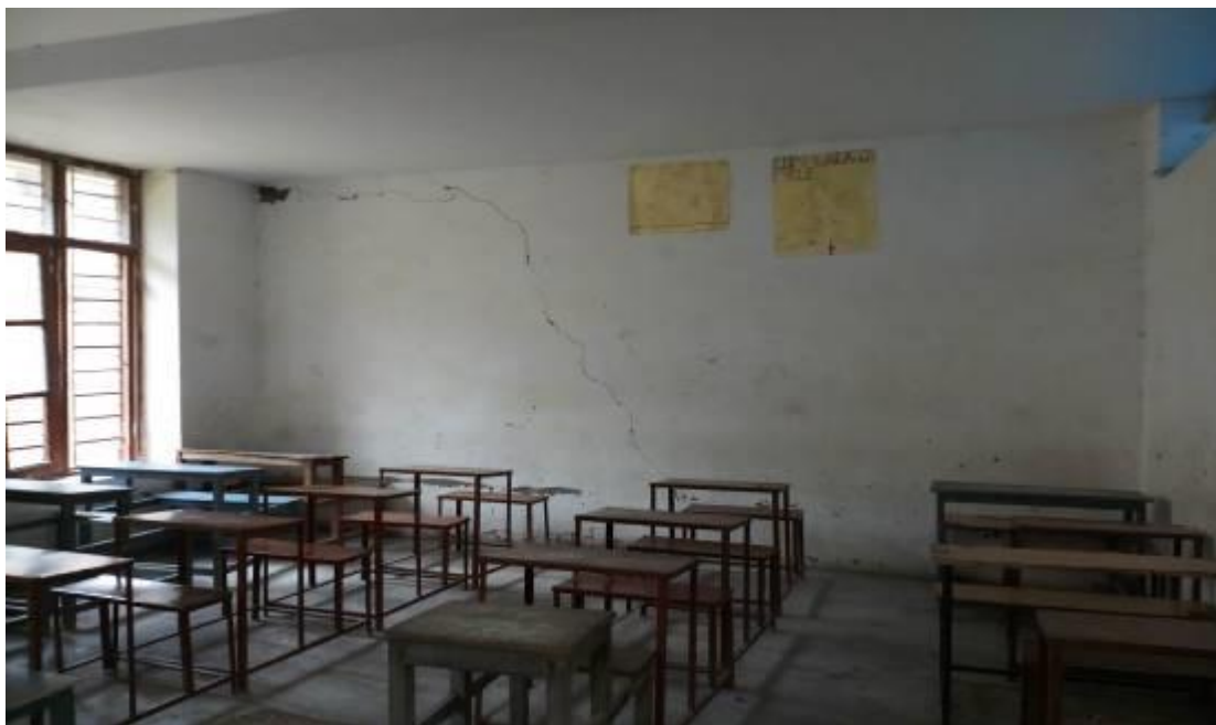
Damaged Block of the school complex
