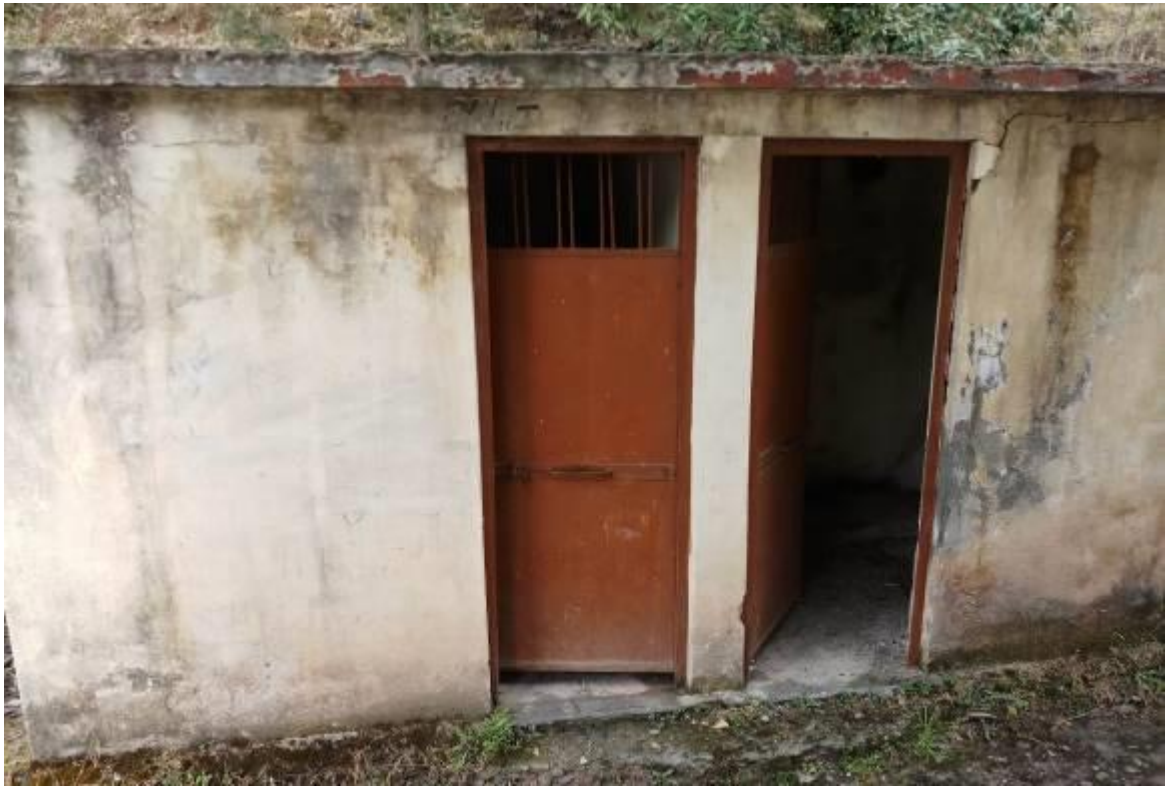
Dilapidated Toilet Block
