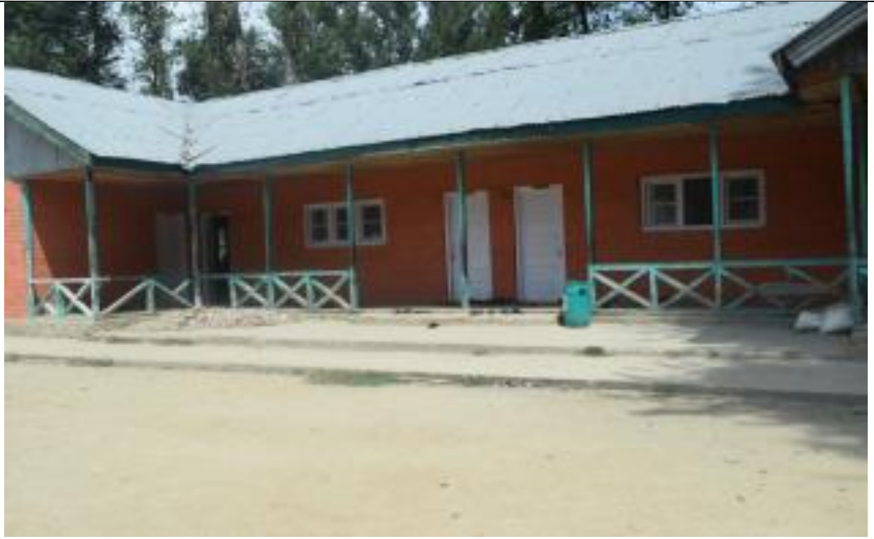
Figure 4-4: flood affected class room block
