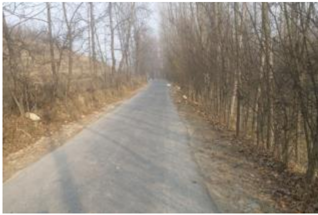
Figure 3-1: Existing road condition
