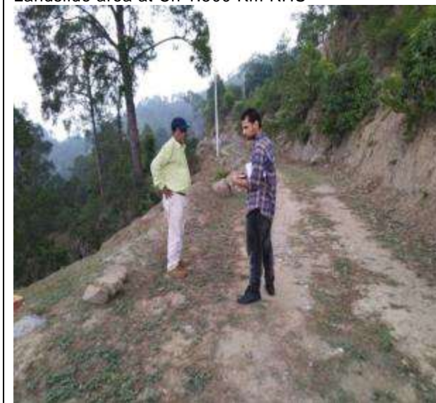
Poor Road Condition at Ch 2.200 km
