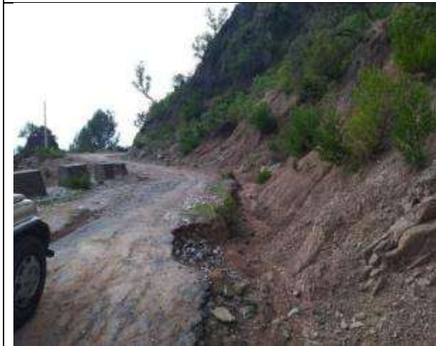
Landslide area at Ch 1.500 Km RHS
