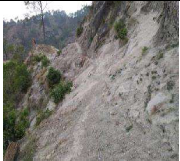
Foot track and Landslide at Ch 7.800 Km
