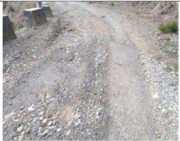
Poor Road Condition at Ch 1.700 Km
