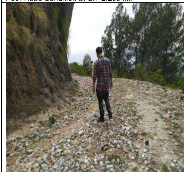
Poor Road condition at 2.700 Km
