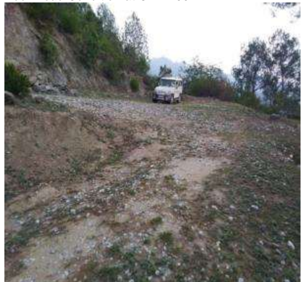
Poor Road Condition at Ch.2.500 km
