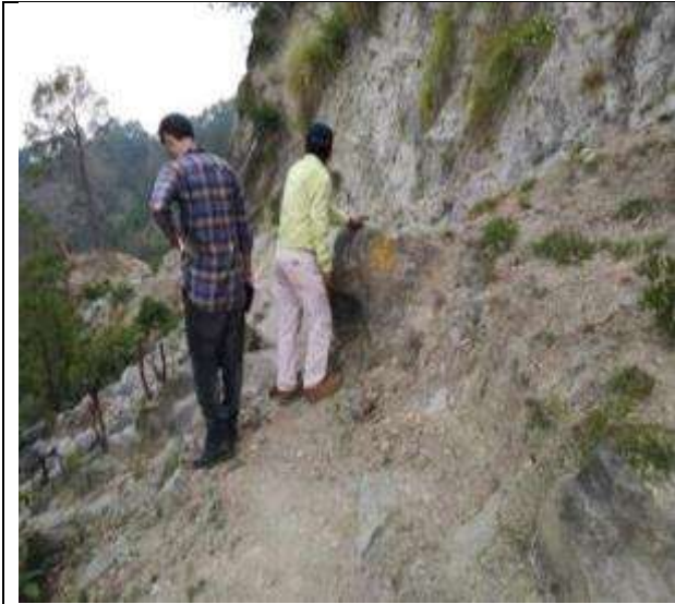
Foot track and Slide area at Ch. 3.700 km
