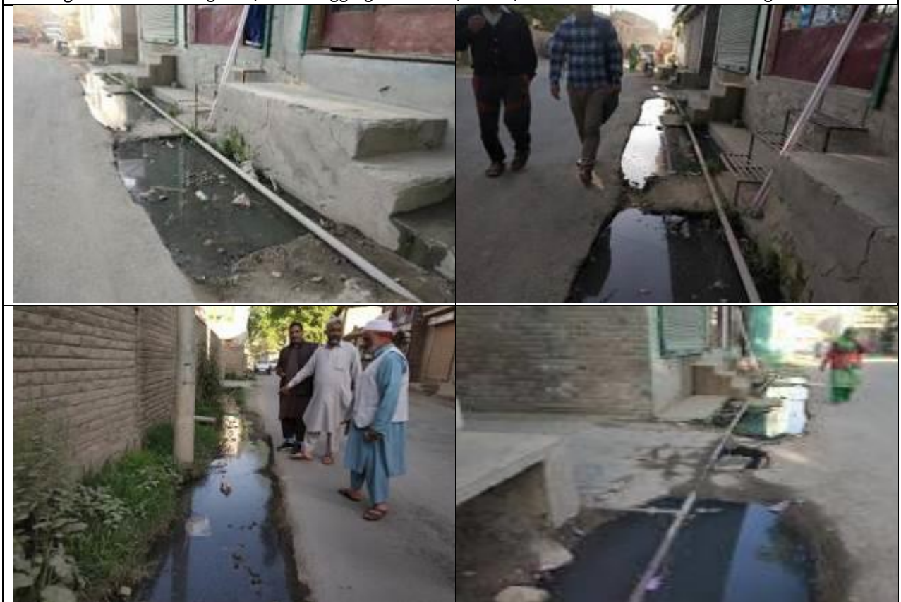
Figure 4-3: Site photos of Padshahi Bagh showing waterlogging and water supply pipelines
