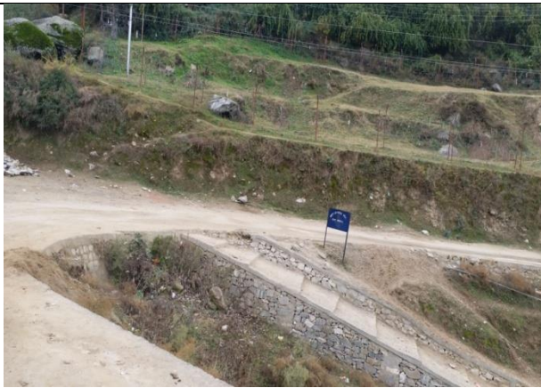
Poor road conditition at Ch 3.800 Km
