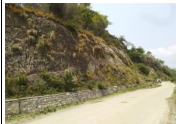
Landslide area (8.200 Km RHS)
