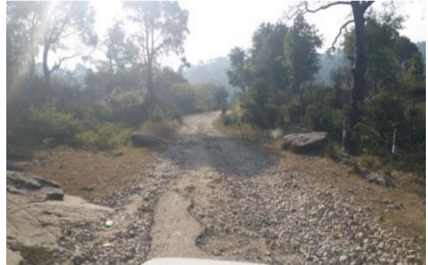
Poor road condition at Ch 9.700 Km
