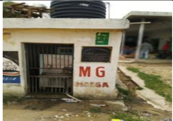
Water tap with tank at Ch 1.950 RHS
