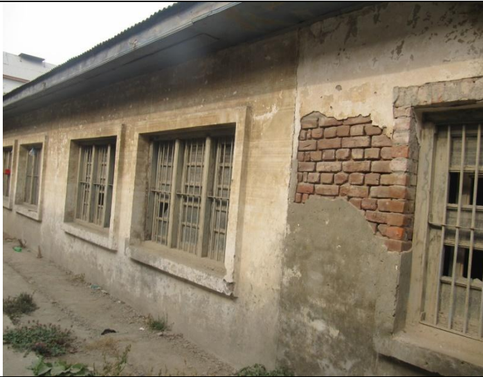
Existing damaged building
