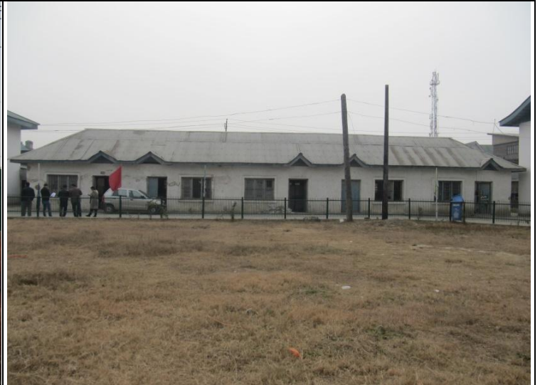
Existing damaged building in school premises
