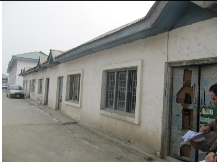
Existing damaged building
