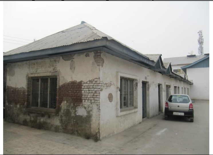
Existing damaged building
