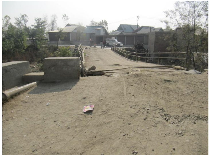
Approach and water supply utilities.
