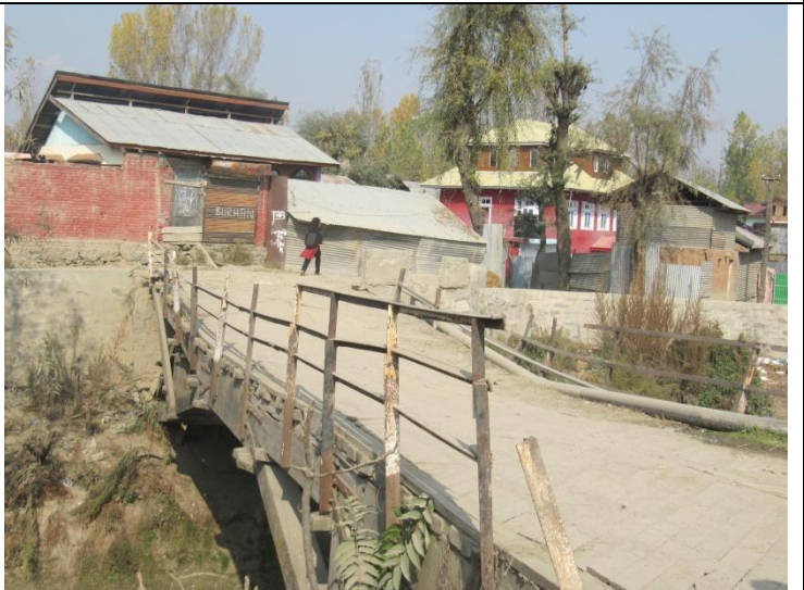
Existing damaged bridge
