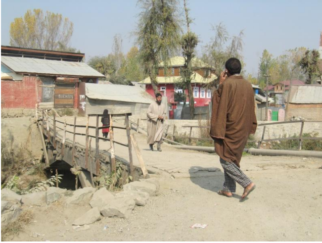
Existing damaged Bridge on NingliNallah
