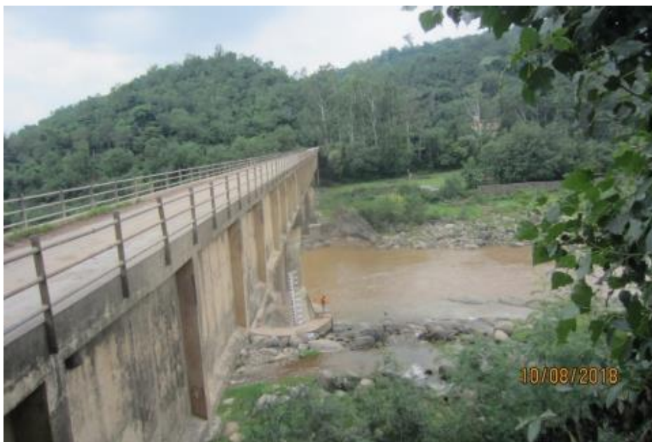
Photo 8.2: Hydrological station on Tawi River at Udhampur
