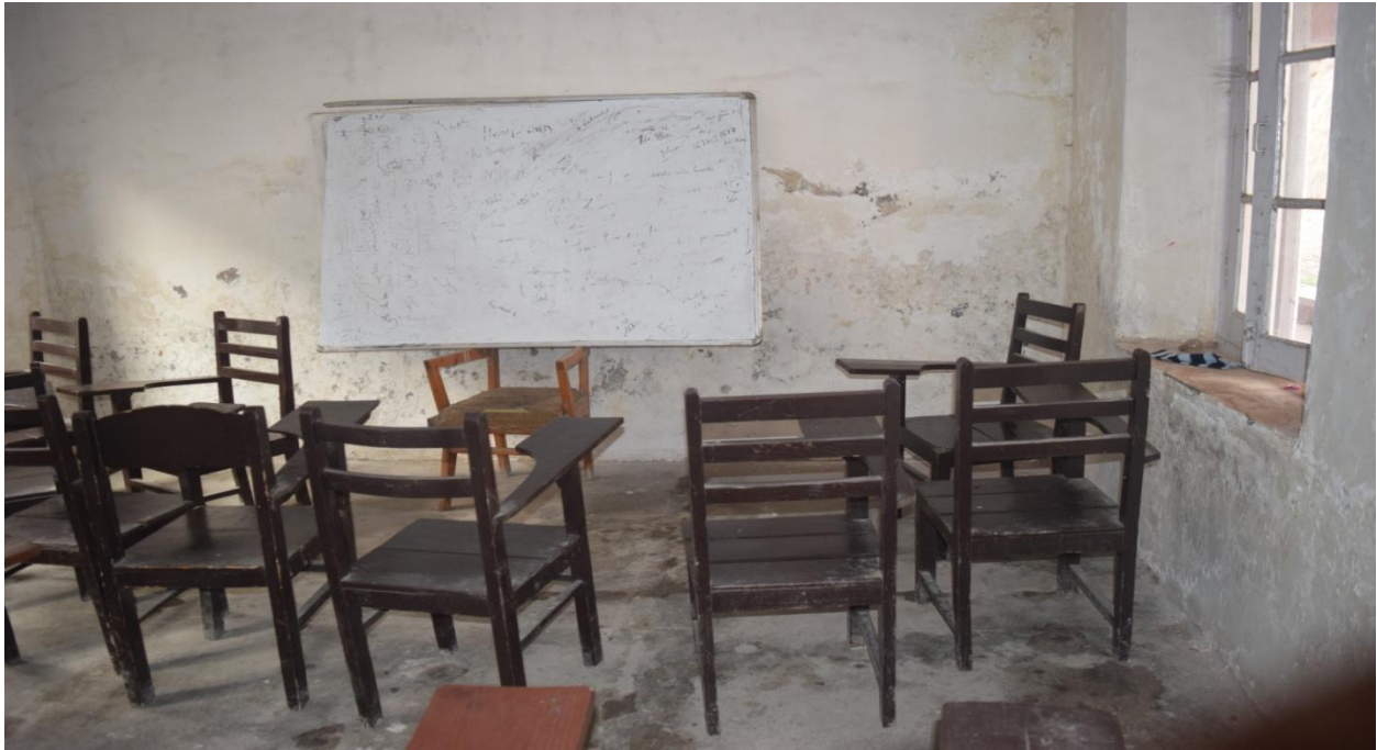
Plate.7. flood affected class rooms
