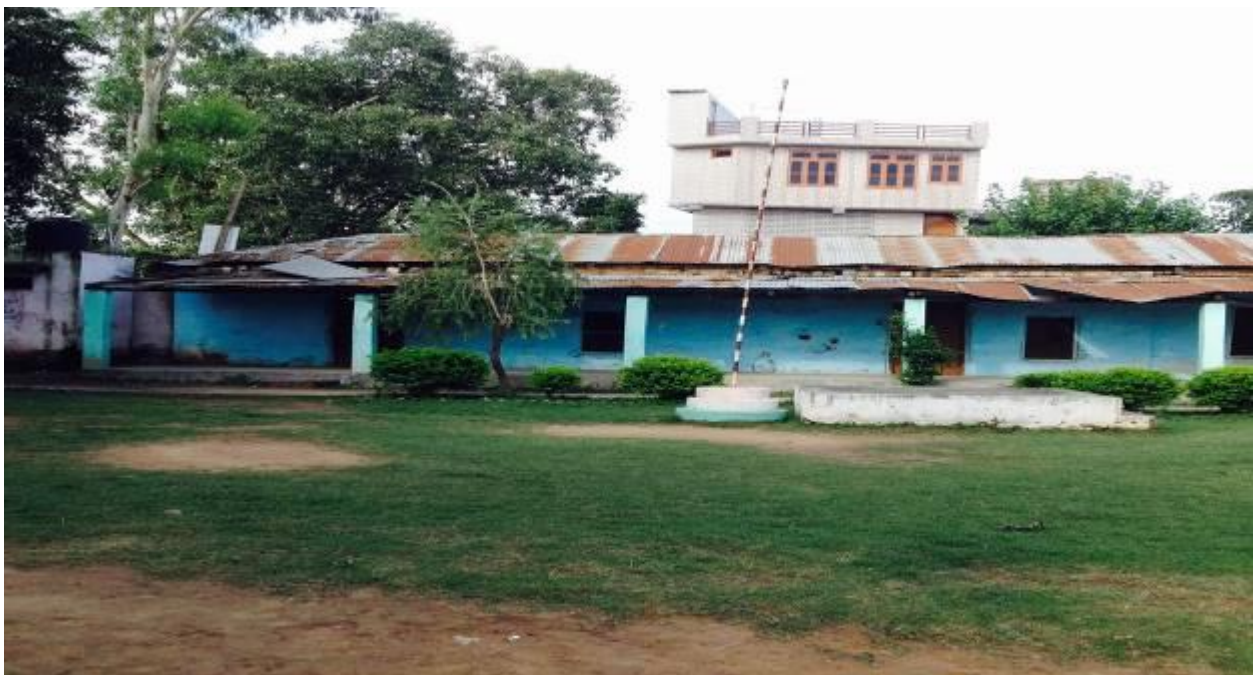
Exterior of Damaged Block
