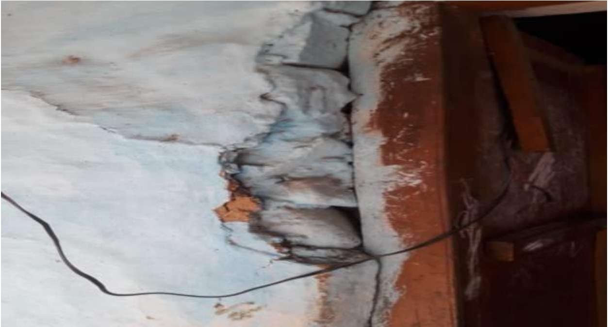
Interior of Damaged Block
