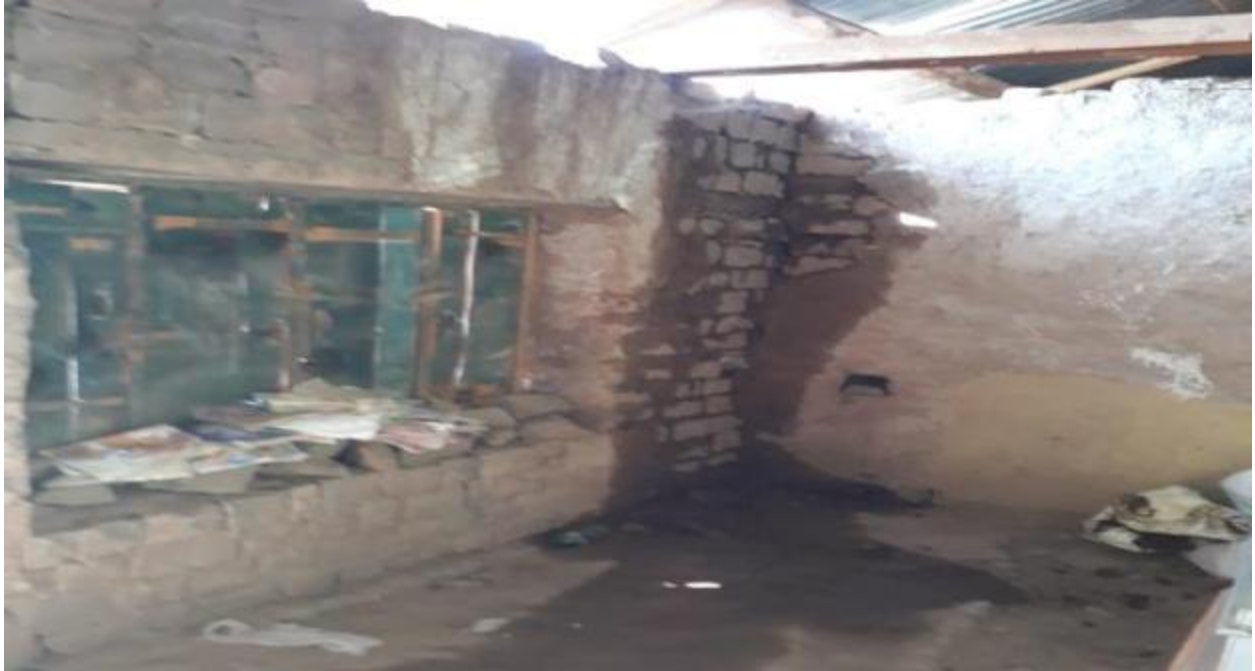
Damaged Interior of the Rooms
