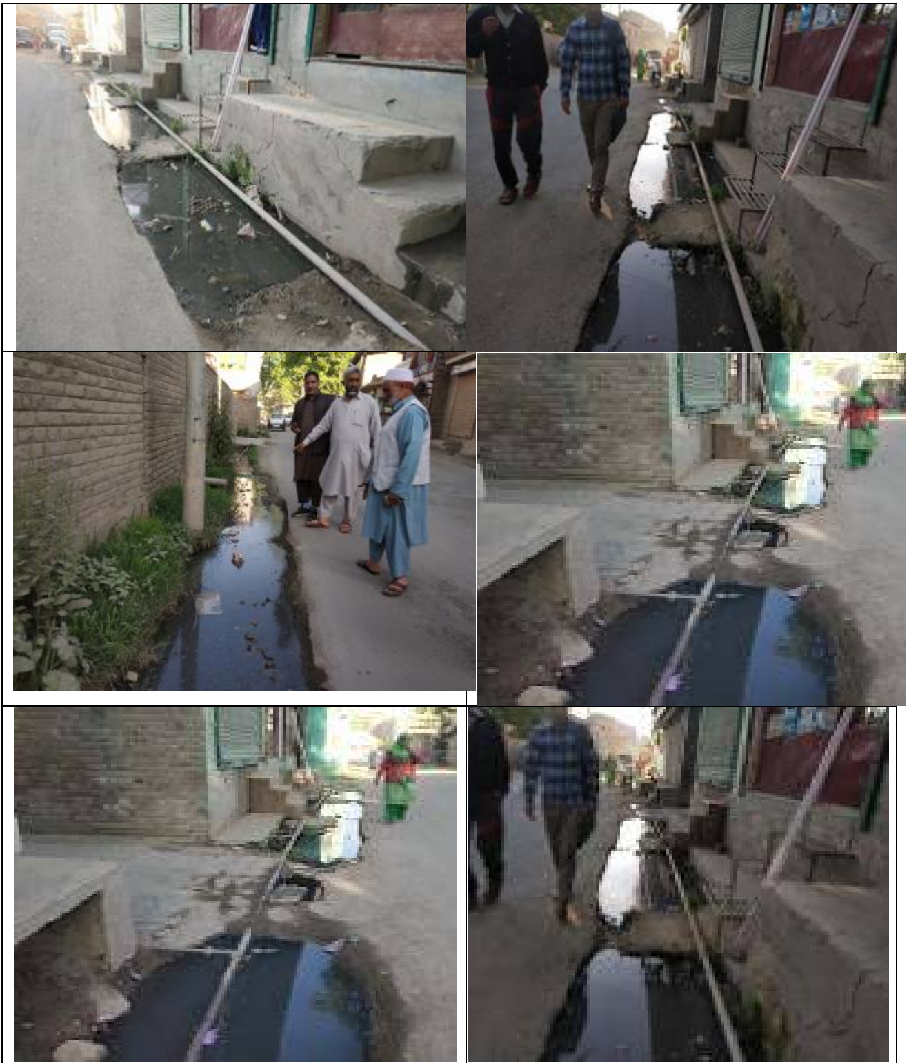
Site photos of Padshahi Bagh showing waterlogging and water supply pipelines passing through stagnant water
