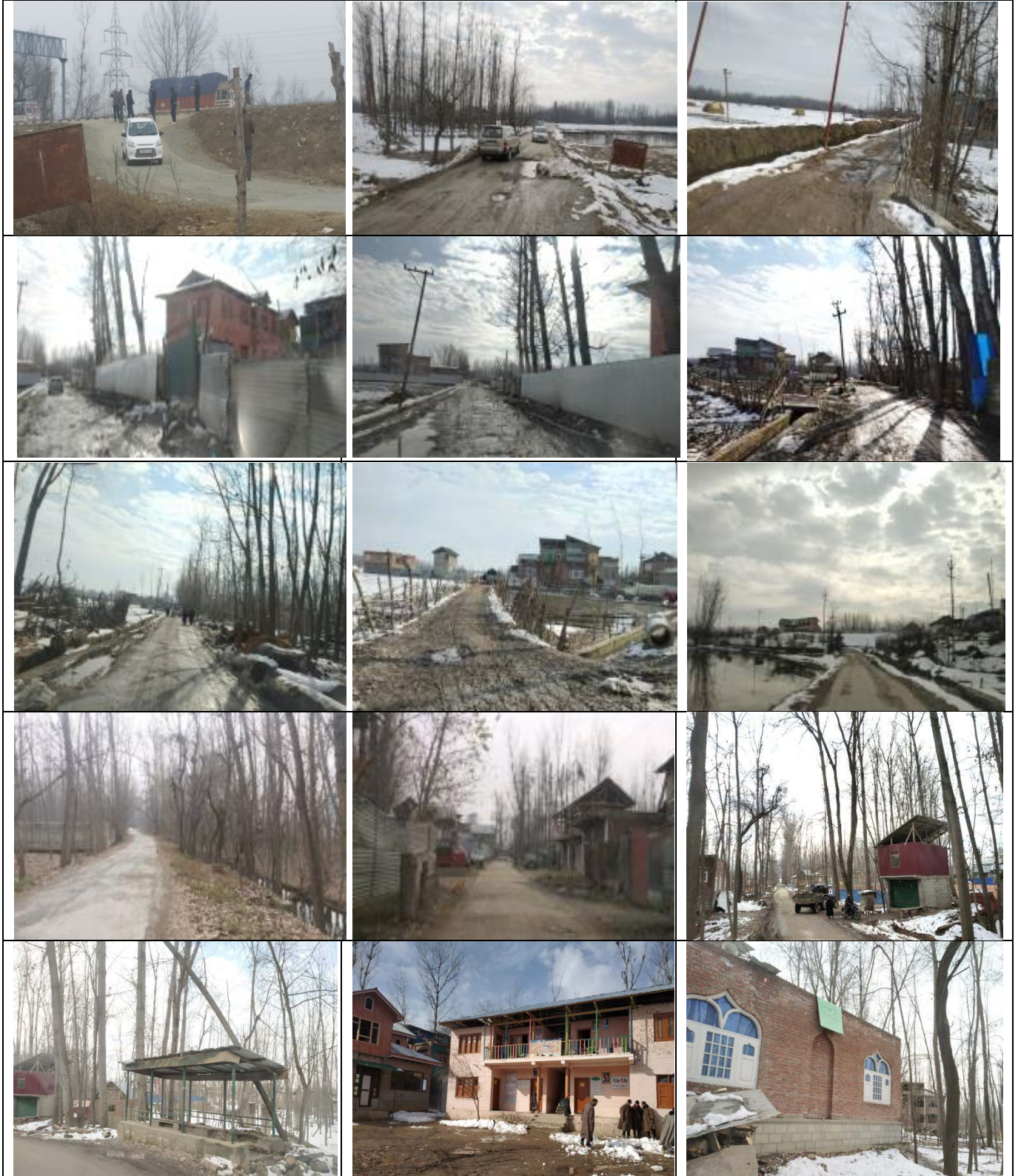
Site photos of Sangam-Khudwani Road showing existing road features which is in highly dilapidated condition. School and religious places are also exists along the road. A bus bay as evident in the above picture is in degraded state.
