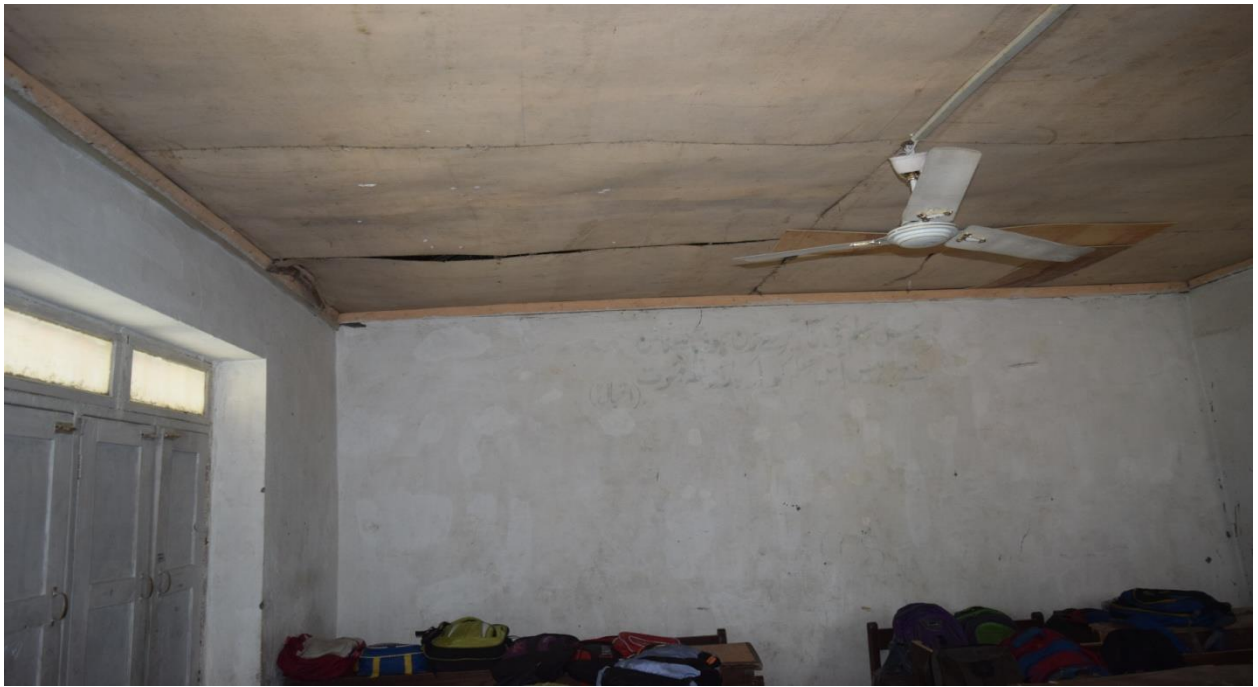
Figure 3-5: Deteriorating condition of false ceiling
