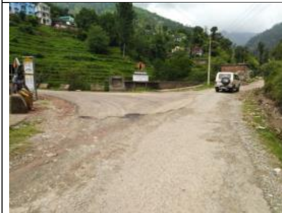
Junction of PMGSY road (left) in the project road at Ch 8.800 Km
