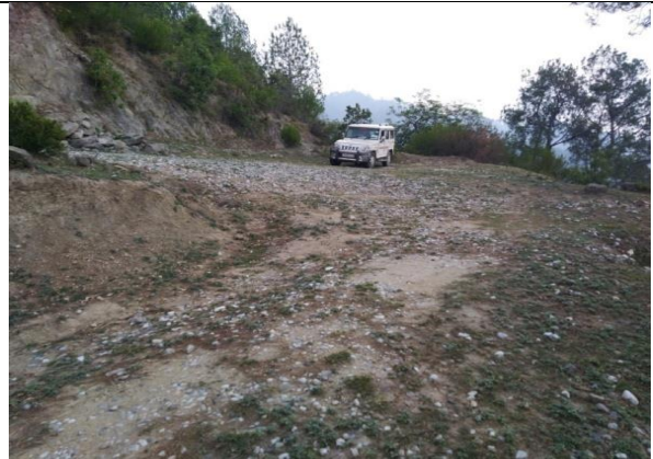
Poor Road condition at Ch 2.500 Km
