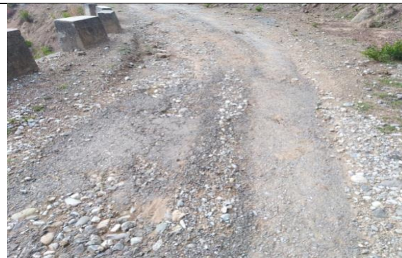
Poor Road condition at Ch 1.700 Km
