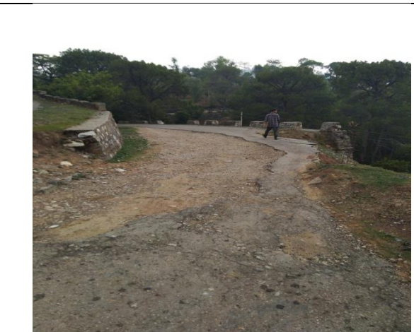
Poor Road conditions at Ch 0..400 Km
