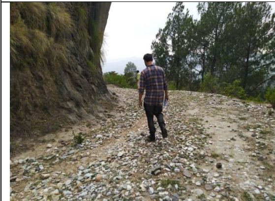
Very poor Road condition at Ch 2.700 Km
