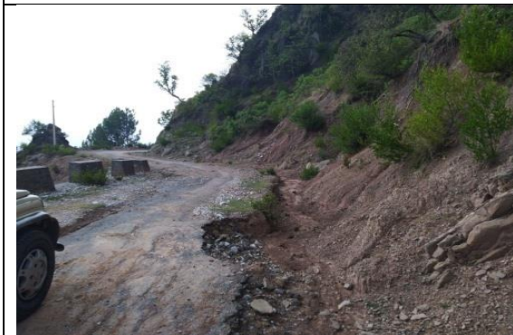
Land slide area at Ch 1.500 Km( RHS)
