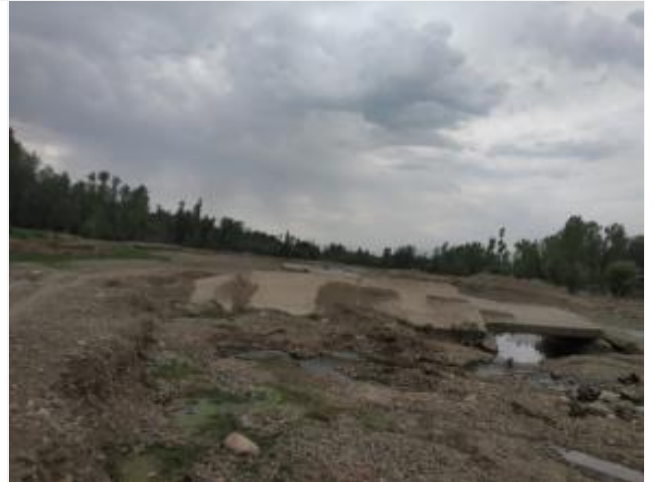
Odds and ends of the damaged bridge (which was washed away during the 2014 floods) near the proposed bridge site downstream.
