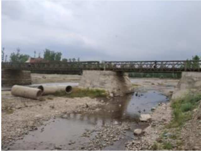
Existing temporary bailey bridge on RHS of the proposed bridge. This temporary was constructed after the 2014 floods and was damaged several times.
