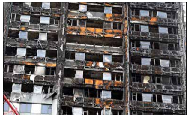
Figure 72 Spread of fire due to use of combustible ACP façade material – Representational picture
