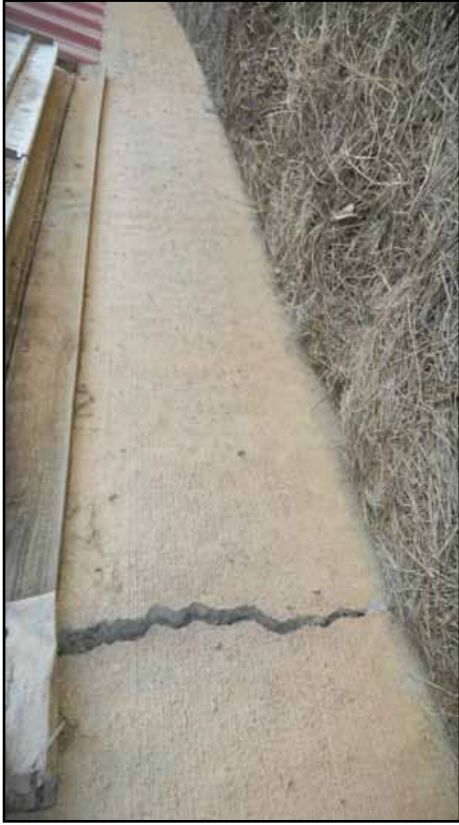
Figure 51a Cracking of Foundation due to rotation/settlement of soil
