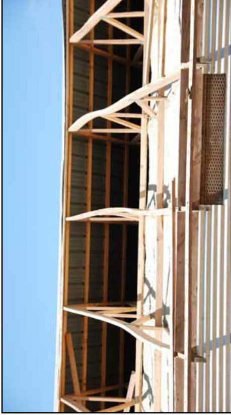
Figure 51b Bracing of trusses is essential to keep trusses vertical and to help carry loads along the length of the house
