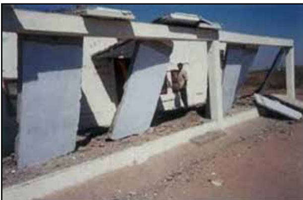
Figure 62 73% of schools made with Precast Construction collapsed or were severely damaged in 2001 Bhuj Earthquake
