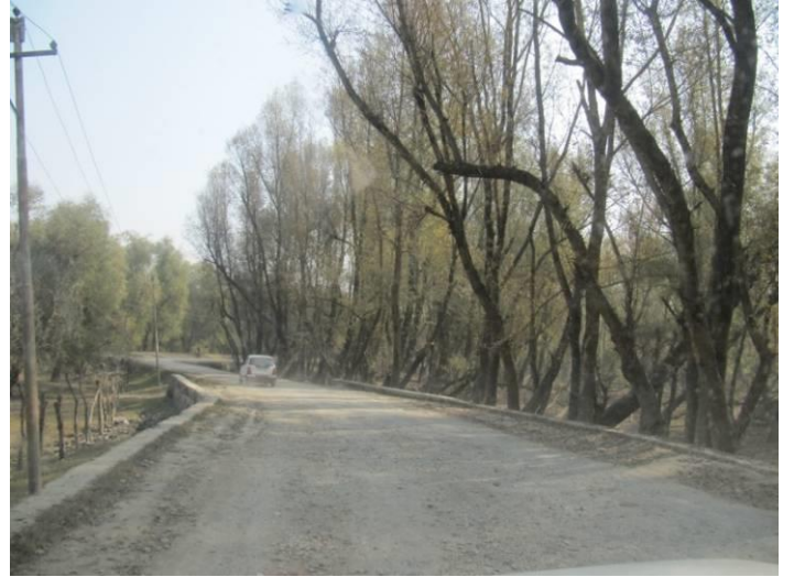
DISTRESSED ROAD IN FLOOD DAMAGE
